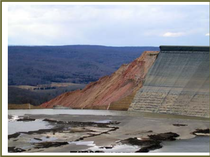
Overtopping ruptures Dam at Taum Sauk Reservoir.
